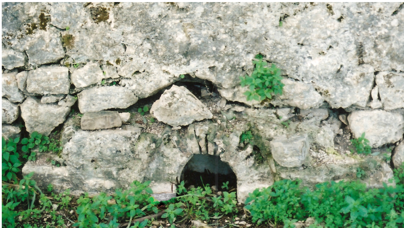
Fig. 227. Vonitsa, Castle, quayside, Koimisi Theotokou sto Limani (old church). Section of masonry.
